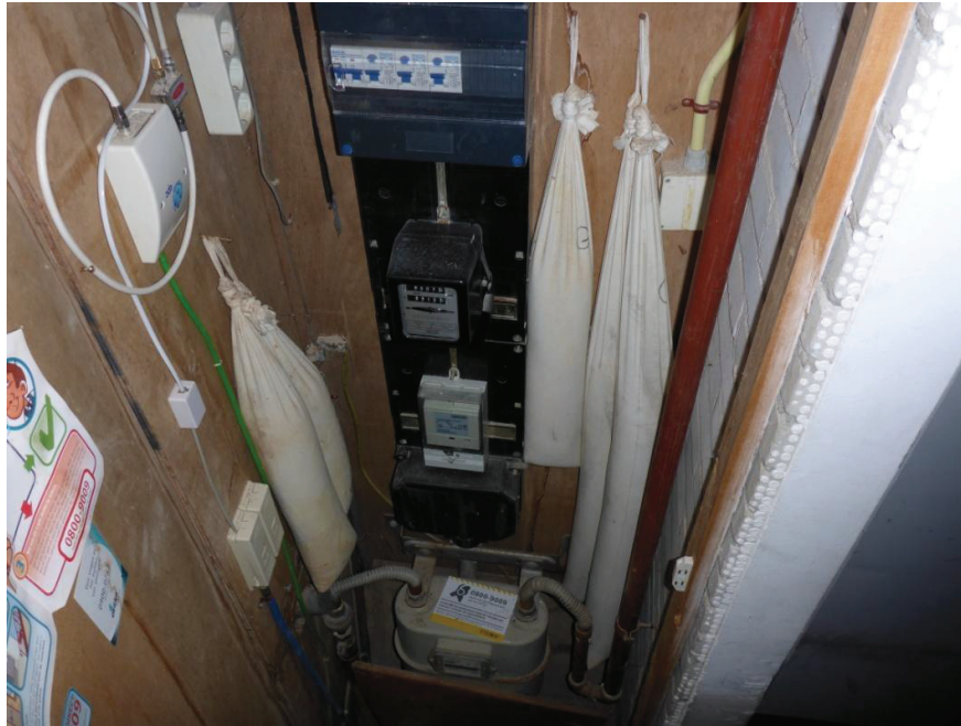
Detailfoto 7: Meterkast in de garage
